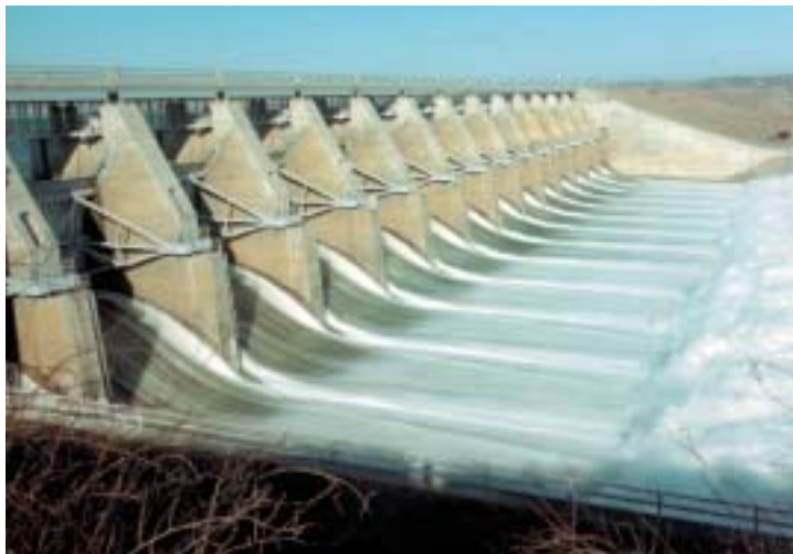
Gavins Point Dam Spillway. View of spillway 29,000 CFS Release. Missouri River. Yankton, South Dakota.
