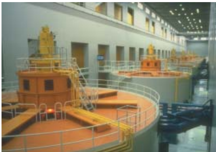
Turbines inside the Bonneville Dam powerhouse, Oregon.
