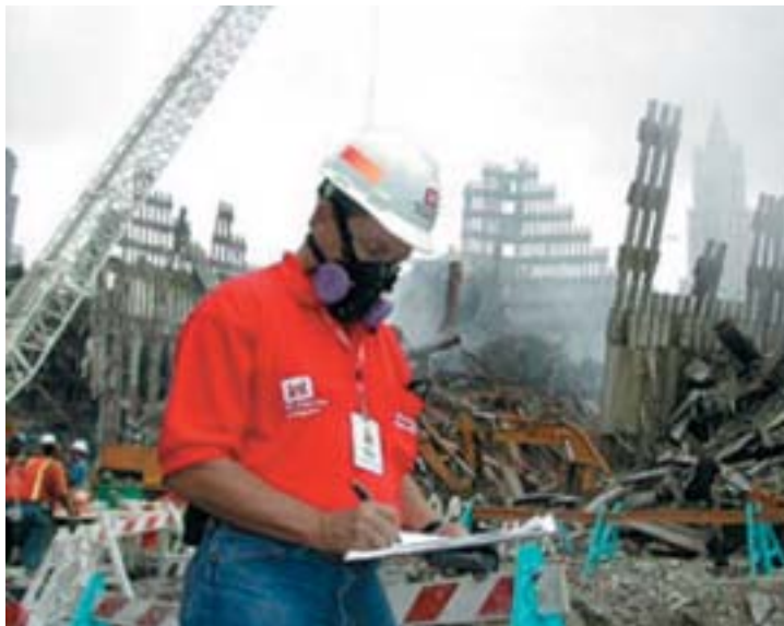
Bob Chapman of the Corps of Engineers Fort Worth District works at "Ground Zero." Personnel of the U.S. Army Corps of Engineers were at Ground Zero just two hours after the hijacked airliners struck the World Trade Center.
