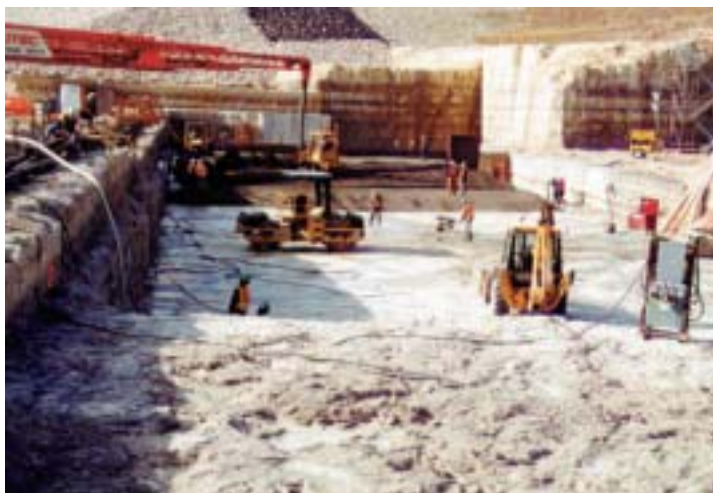
Workers place roller-compacted concrete beneath the Table Rock Auxillary Gated Spillway in late January 2001. Approximately 7,000 cubic yards were placed over a period of seven days.
