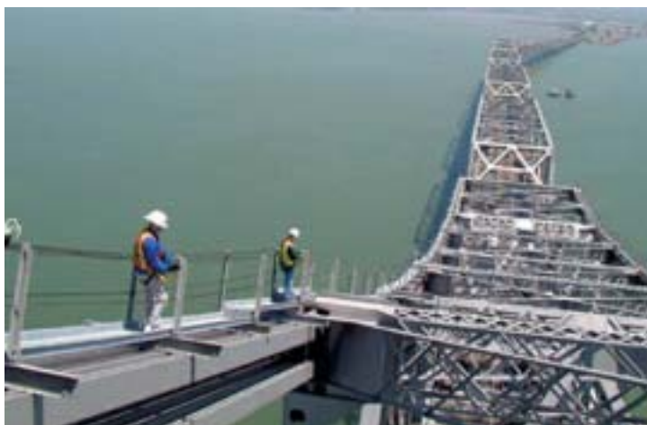
The Corps review team takes a dramatic trek on the San Francisco-Oakland Bay Bridge to get a first-hand look at its construction as part of its recent safety assessment.
